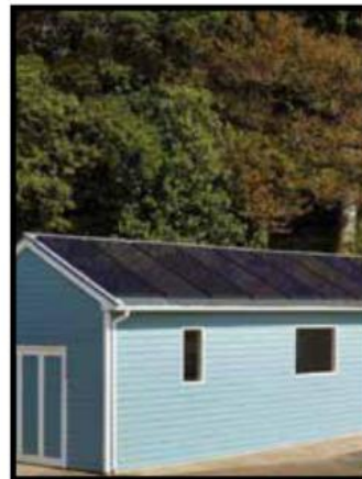
Often, covering a whole gable is the best way to relate to the general shape of a roof
