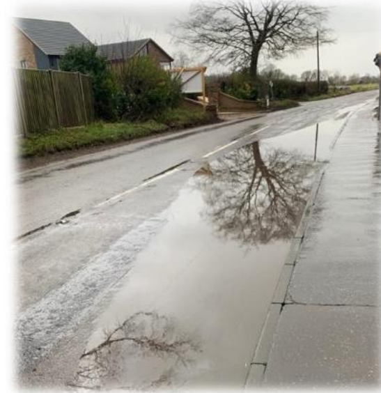
Flooding, A1064, Pound Lane and Marsh Road, January 2021
